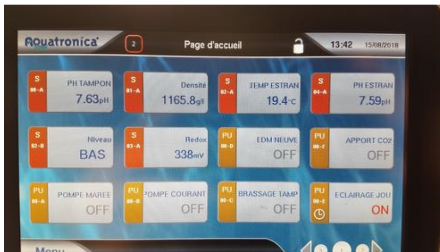
Figure 7: Aquatronica control module
